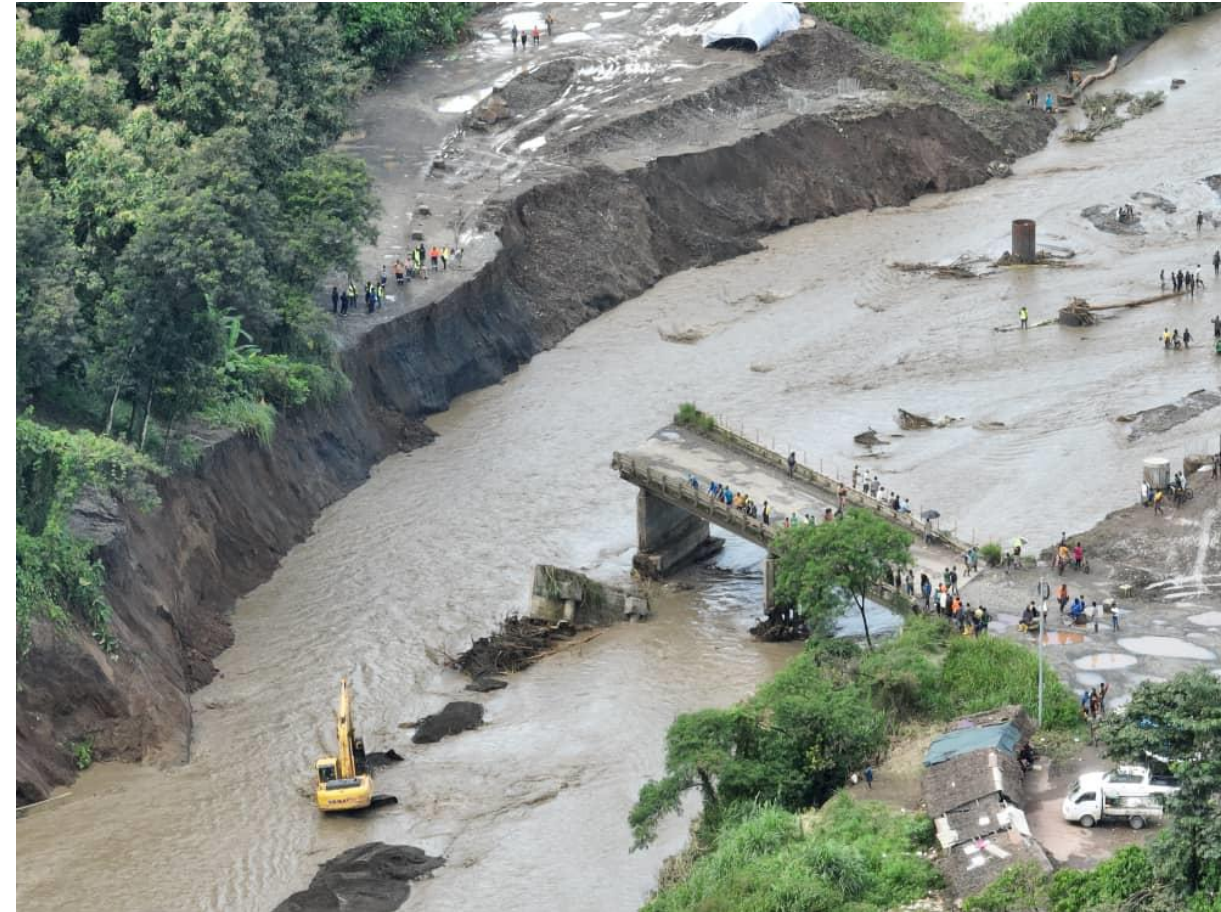
Approx. 70 years Bridge has collapsed-2024
