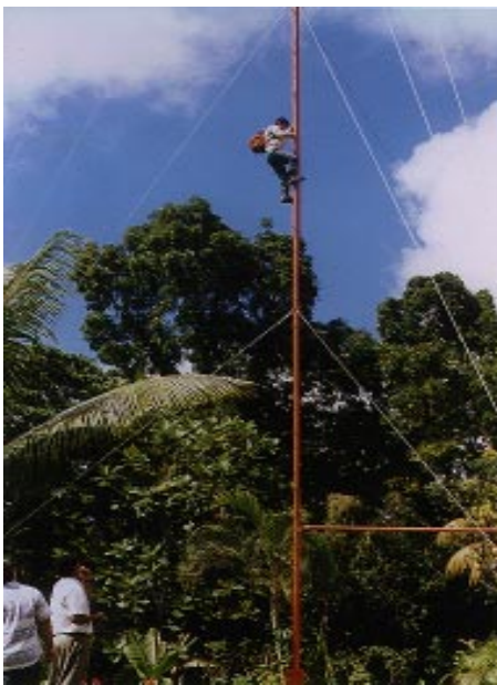
Figure 1: The antenna mast is 25m in height to guarantee a free view to the horizon above the trees.
