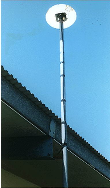
Figure 2: Antenna of the base station installed at FEA, Lautoka. The cable is connected with the Base Station
