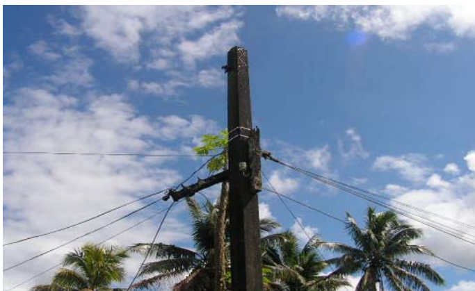
Figure 3: An example of a defect captured in the field. Cross arm of the power pole pictured above is broken and should be replaced.
