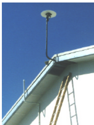
GPS antenna of Solomon Islands Electricity Authority
